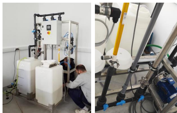
Figure 1: Presentation of the UF system installed (left) and the three membranes examined (right).
