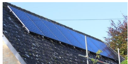
Figure 2: System 2 Panels Top: SE & SW-facing; Lower: NE-facing
