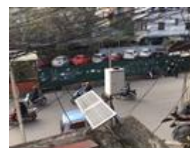
Cairnet station installed in Hanoi
